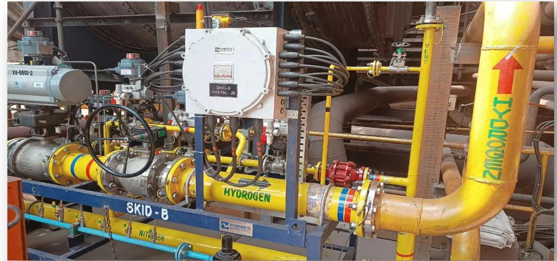
Hydrogen injection in blast Furnace
