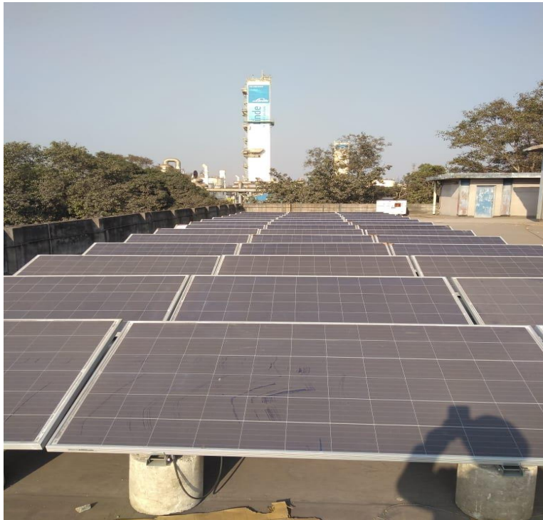
Roof Top Solar
