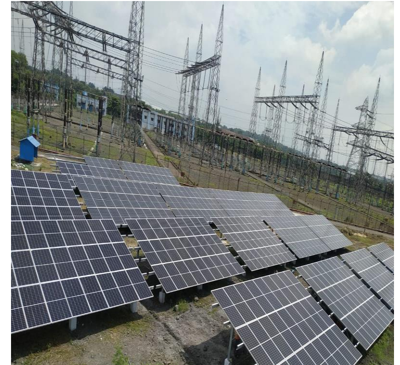
Ground Mounted Solar
